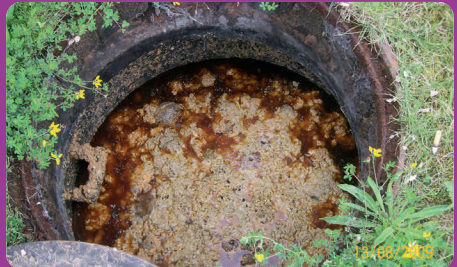
Fat building up in a manhole.
