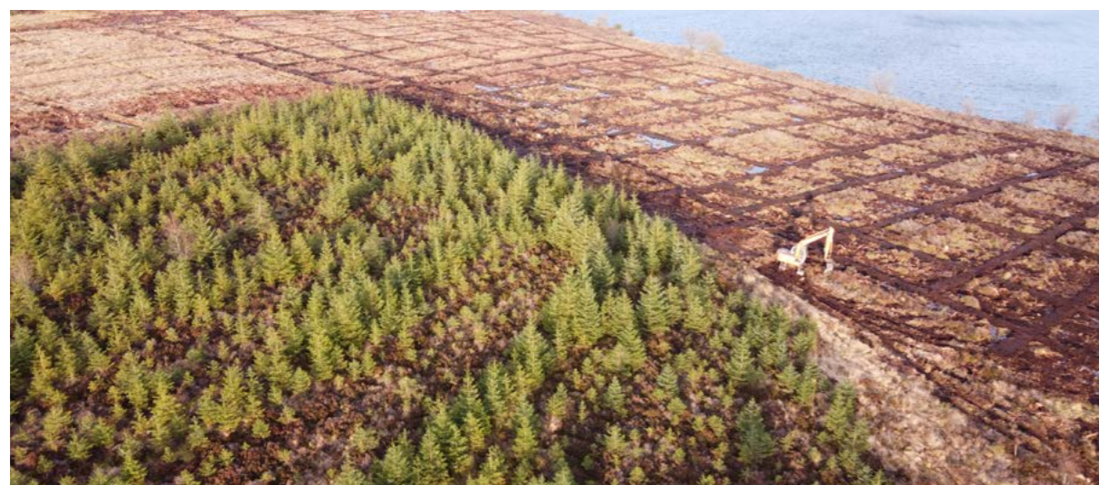
Forestry operations to fell trees adjacent to Lough Bradan reservoir, County Down.
