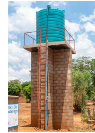
Water tank installed to ease water challenges, Kawinga Health Centre, Machinga, Malawi. Photo credit WaterAid/Francis Chipanda.
