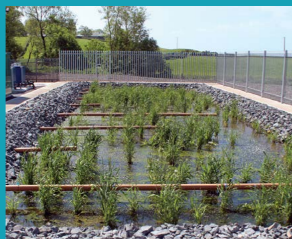
Aerated reed bed growth at Loughries wastewater treatment works, Newtownards, County Down.
