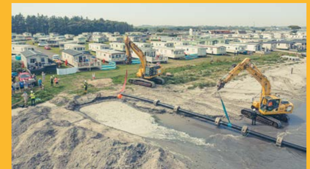
The long sea outfall during installation off the coast, adjacent to a caravan park at Ballyferris, County Down.
