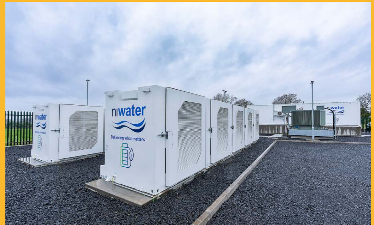
NI Water's state-of-the-art battery energy storage system at Dunore Point, County Antrim.
