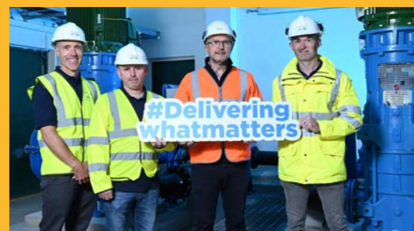
NI Water staff and contractor with the energy efficient pumps installed at Ballygomartin water pumping station, County Antrim.
