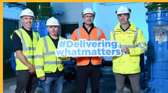
NI Water staff and contractor with the energy efficient pumps installed at Ballygomartin water pumping station, County Antrim.
