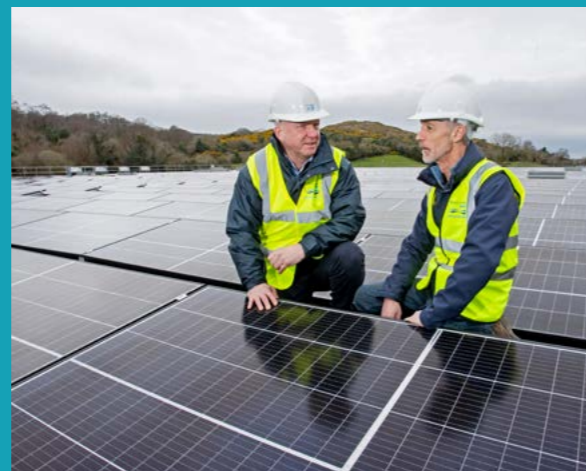
Solar installation at Drumaroad water treatment works, Castlewellan, County Down.
